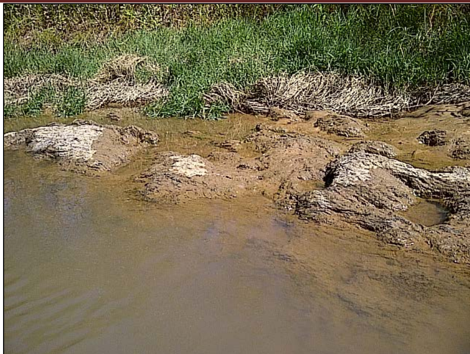
Figure A-29 Left Bank of River Consists of Bed Rock at Abstraction Works Position
